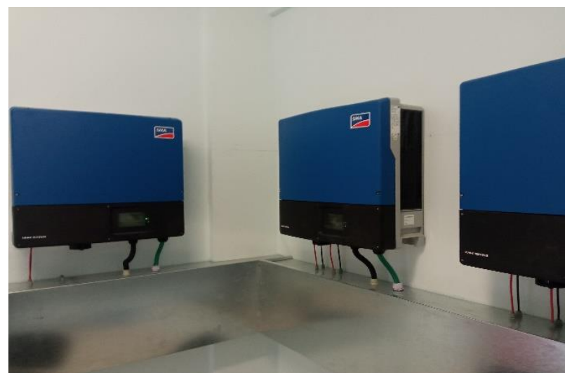
Solar system control room
