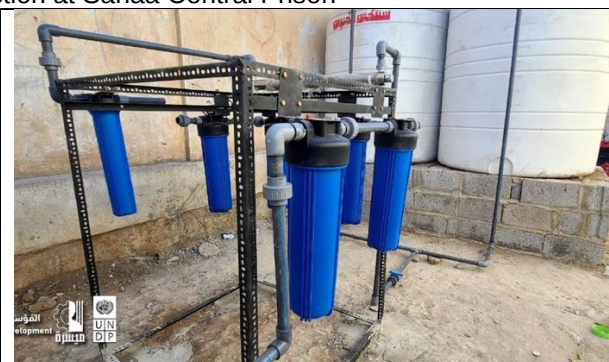
Rainwater harvesting unit at Sanaa Central Prison
