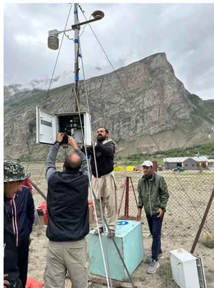
Figure 11: Installation AWS at Askole
