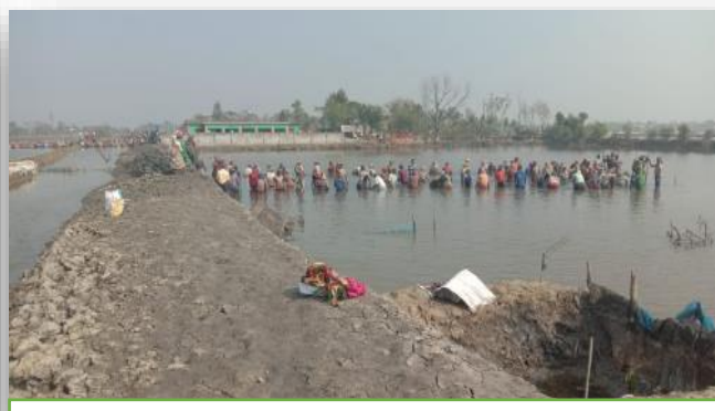
Photo 4: Earthen Road construction is almost completed under Cash for work in Shyamnagar Sub-district. District: Satkhira
