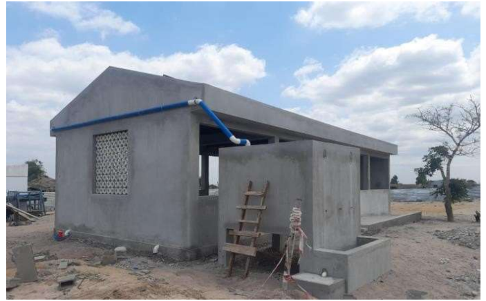
Isometric view of market with rain water collecting tank at finishing level in Mutua
