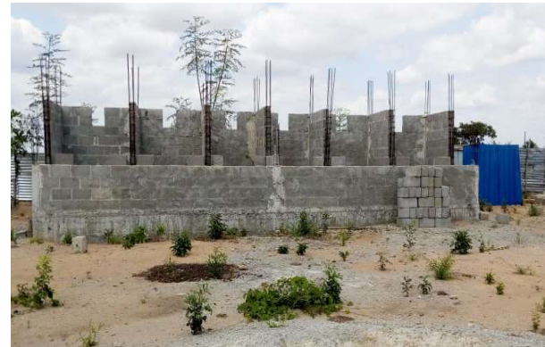
Front view of a toilet construction at lintel level in Guara Gura Buzi
