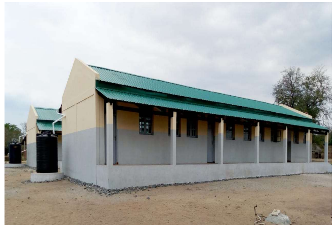
School block-1 is under construction at roof level in Heua, lot2, Chibabava district.
