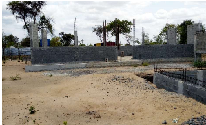
Front view of the market under construction in raising wall in Guara Gura Buzi
