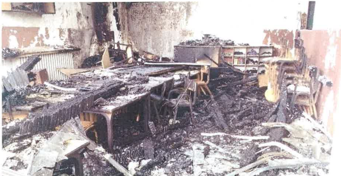
A classroom at the April 8 th Kindergarten after fire destroyed the facility on 28 February 2017
